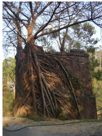
Fig. 7 – Tree attached to Pier 6.
