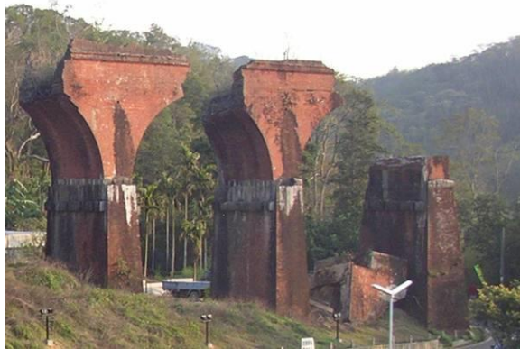
Fig. 4 - The broken brick arcade in north side, the arch spandrel of pier 4 was collapsed by 1999 Chi-Chi earthquake.
