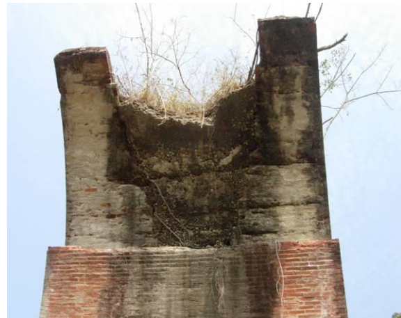
Fig. 5 - The archivolt of brick arcade was drop out.
