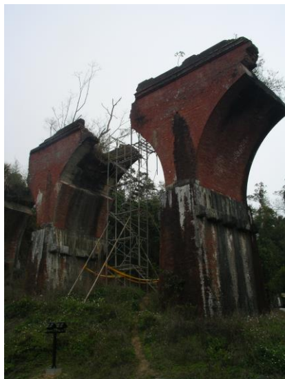
Fig. 6 - Accumulation of soluble salts of Pier 1 and Pier 2
